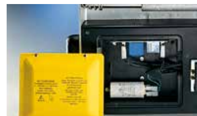
Sealed electrical enclosure
