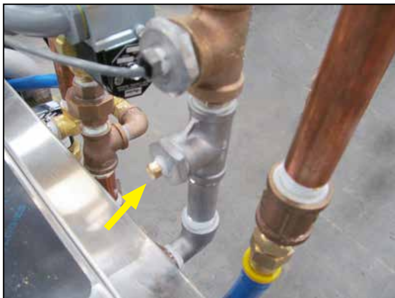
Fig. 13 - Rinse Aid Injection Point
