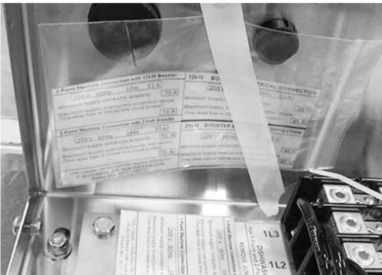
Fig.17 - The 2-point data plate is located in a plastic bag next to the terminal block.
